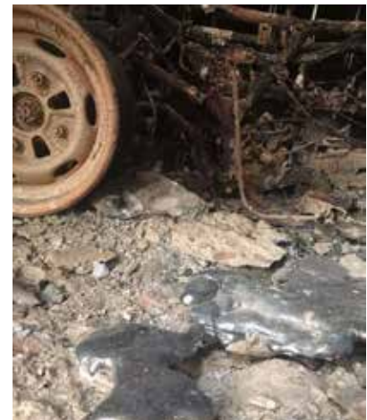
Damage caused by the fire inside the sheds.
